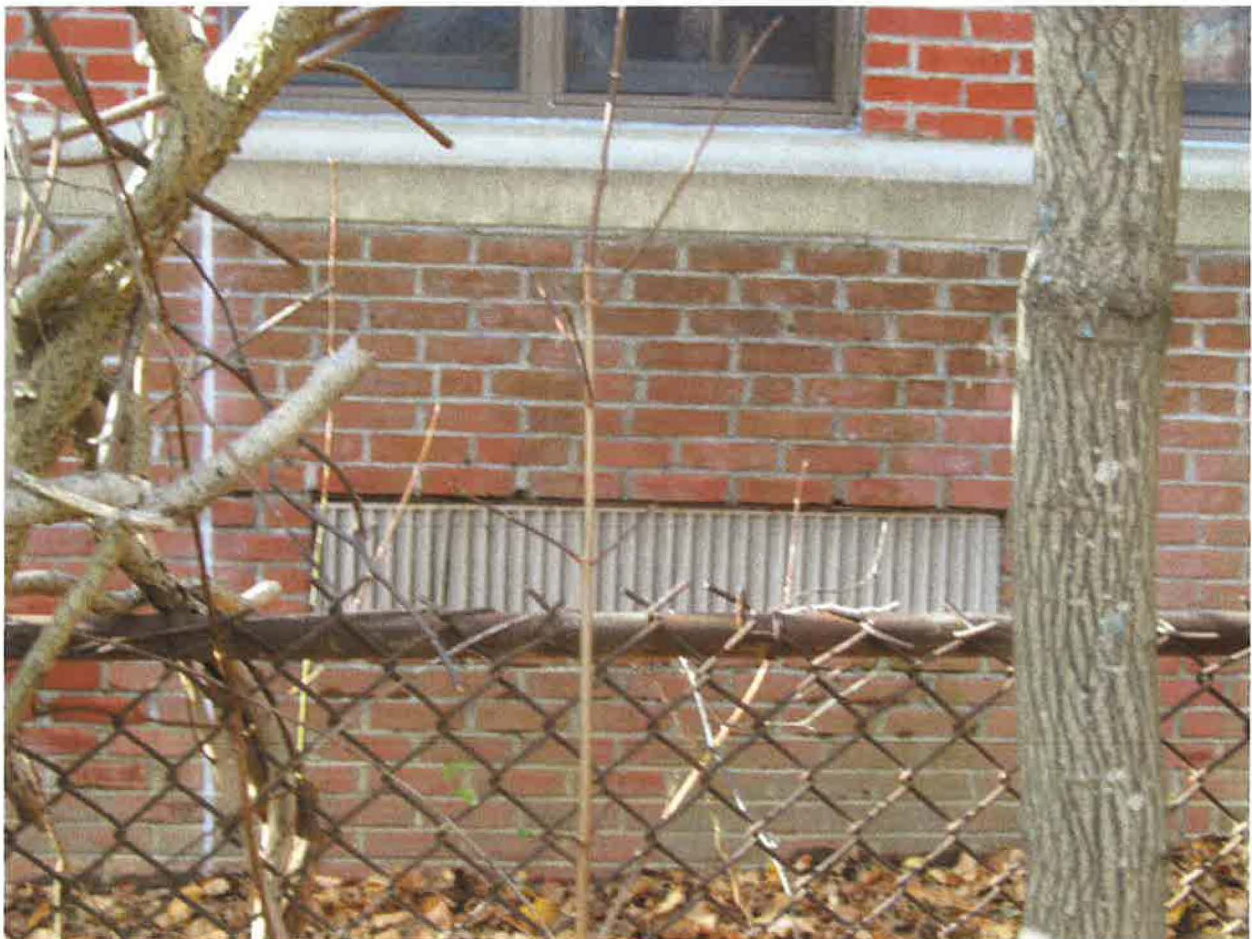
Note lead sleeves at perimeter for bolting flood boards
